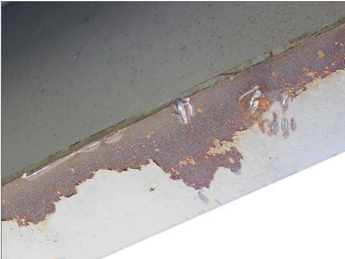
SPAN 1 BEAM 5 - IMPACT DAMAGE OVERVIEW
