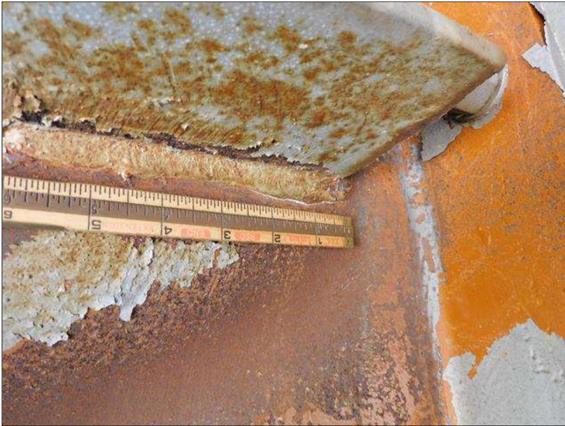
Span 1 Bay 1: IMPACT DAMAGE 4/2022 - INT. DIAPHRAGM 2, BEAM 1 CONNECTION, BOTTOM WELD - 4"L CRACK AT TOE OF WELD (PAR)
