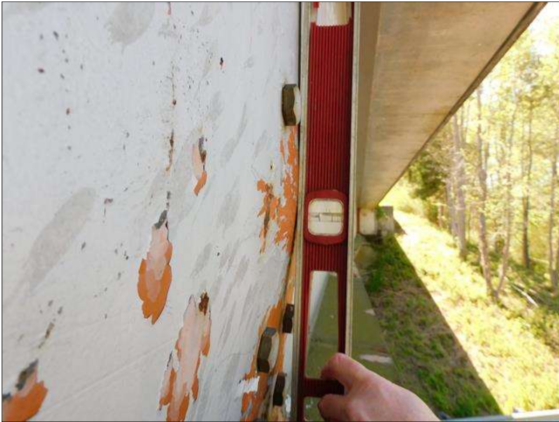
Span 1 Beam 1: IMPACT DAMAGE 4/2022 - 24" DIAMETER SECTION OF WEB DEFLECTED 1-1/4" TO THE NORTH AT INT. DIAPHRAGM 3 CONNECTION (PAR)
