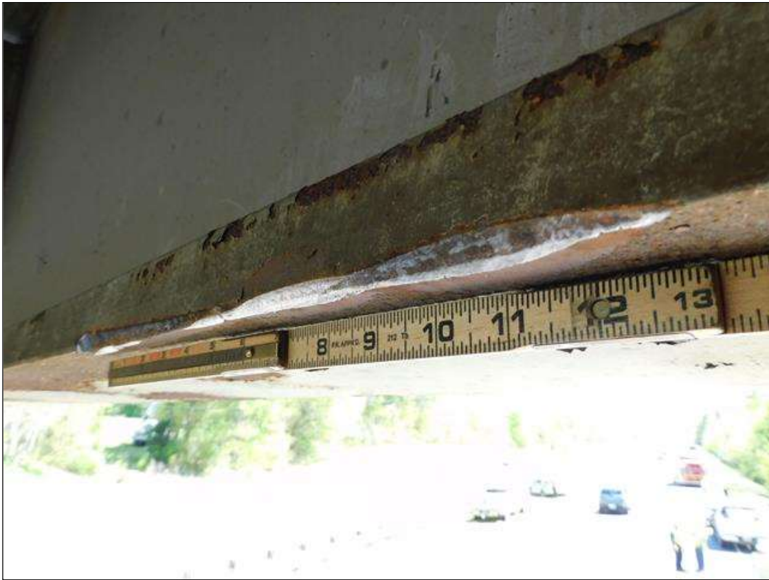
Span 1 Beam 5: IMPACT DAMAGE 4/2022: 13"L x 1/2"W x 1/4"D INDENTION ON NORTH EDGE OF BOTTOM FLANGE AT 57' FROM END BENT 1 BEARING
