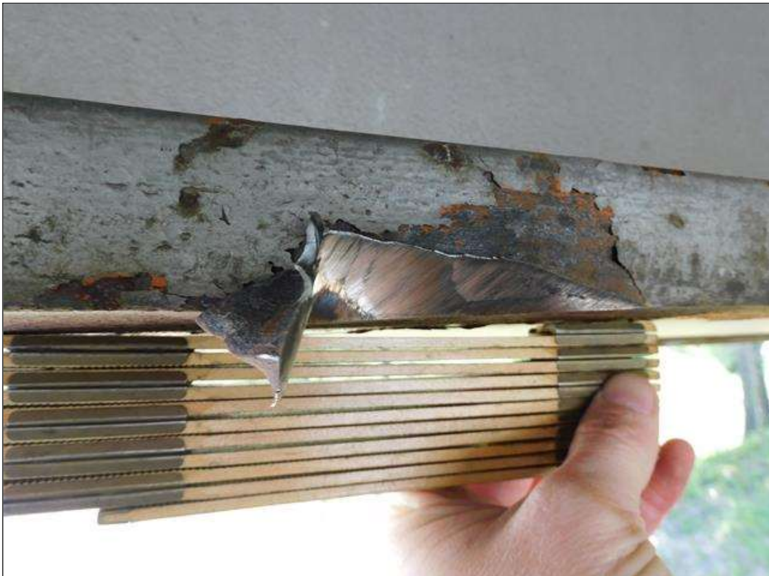
Span 1 Beam 4: IMPACT DAMAGE 4/2022: 3-1/2"L GOUGE UP TO 5/8"D ON NORTH EDGE OF BOTTOM FLANGE - LOCATED 56' FROM END BENT 1 BEARING (PAR)
