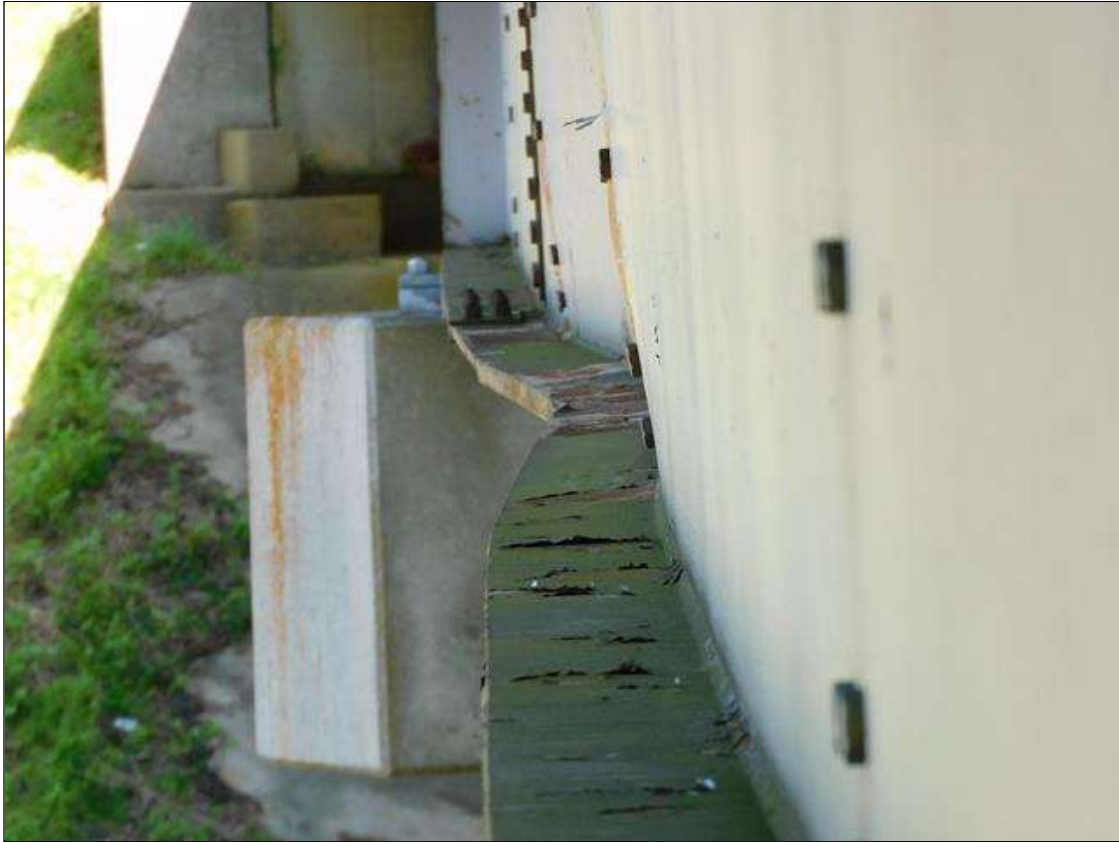
Span 1 Beam 1: IMPACT DAMAGE 4/2022: 23LF OF BEAM OUT OF PLUMB TO THE SOUTH UP TO 4-3/4" - MAX DEFLECTION AT 55' FROM END BENT 1 BEARING - SECTION LOCATED BETWEEN INT. DIAPHRAGMS 2 AND 3 (PAR)
