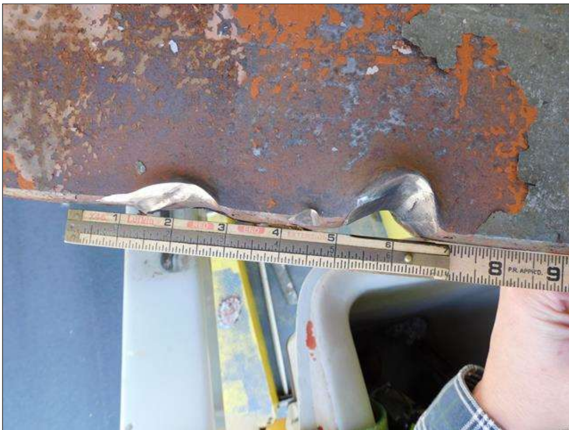
Span 1 Beam 1: IMPACT DAMAGE 4/2022: (2) INDENTIONS UP TO 1-1/2"W x 5/8"D ON NORTH EDGE OF BOTTOM FLANGE AT 55' FROM END BENT 1 BEARING (PAR)
