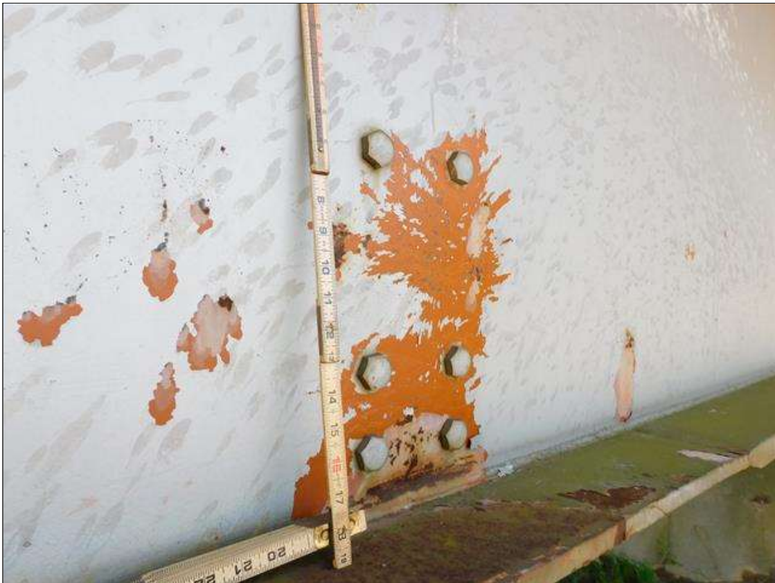
Span 1 Beam 1: IMPACT DAMAGE 4/2022 - 24" DIAMETER SECTION OF WEB DEFLECTED 1-1/4" TO THE NORTH AT INT. DIAPHRAGM 3 CONNECTION (PAR)
