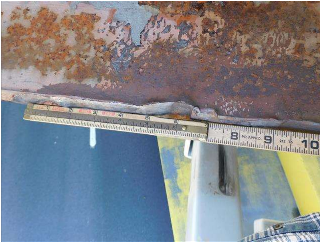
Span 1 Beam 1: IMPACT DAMAGE 4/2022: INDENTIONS UP TO 1-1/2"W x 1/4"D SCATTERED ALONG 10" SECTION OF BOTTOM FLANGE ON NORTH SIDE - LOCATED 56' FROM END BENT 1 BEARING (PAR)
