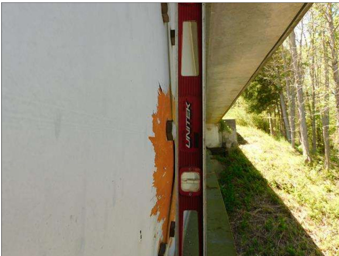
Span 1 Beam 1: IMPACT DAMAGE 4/2022 - 24" DIAMETER SECTION OF WEB DEFLECTED 1-1/4" TO THE NORTH AT INT. DIAPHRAGM 2 CONNECTION (PAR)
