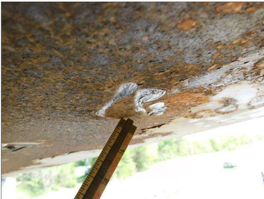
Span 1 Beam 5: IMPACT DAMAGE 4/2022: (3) GOUGES UP TO 2"L x 1/2"W x 1/16"D ON BOTTOM SIDE OF BOTTOM FLANGE - LOCATED 55'-6" FROM END BENT 1 BEARING
