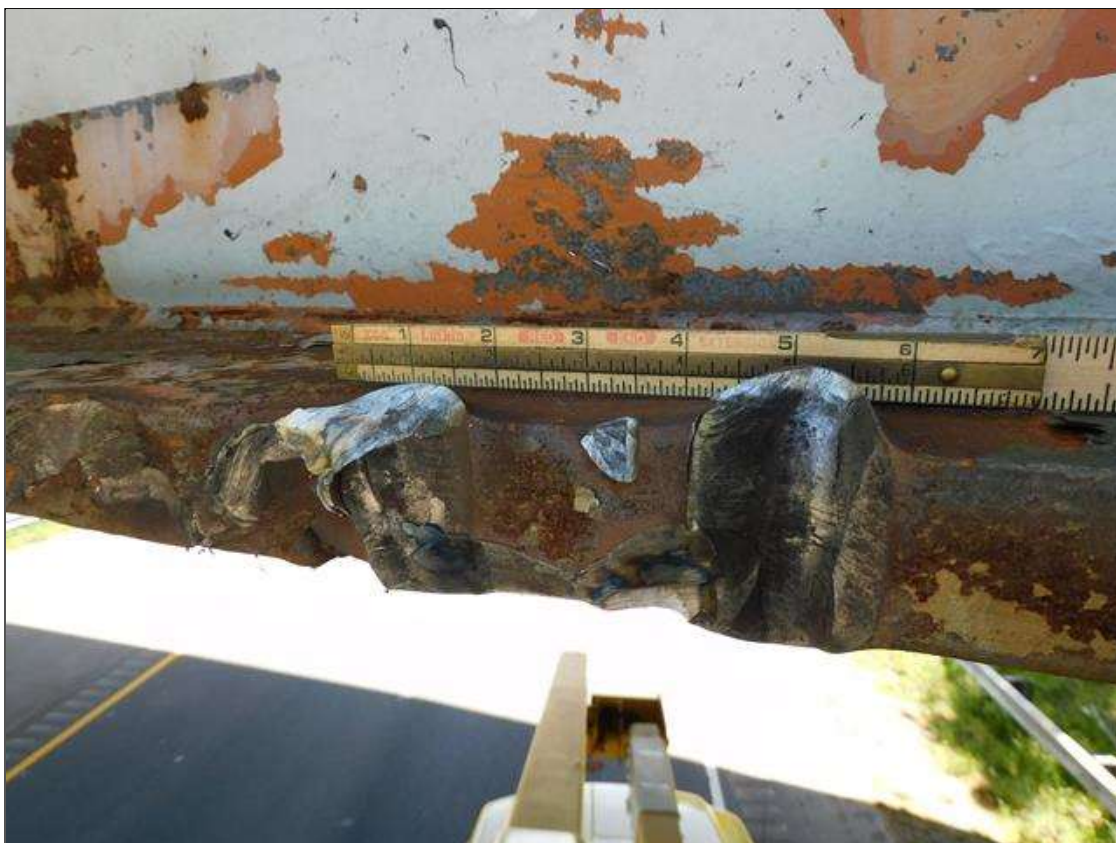
Span 1 Beam 1: IMPACT DAMAGE 4/2022: (2) INDENTIONS UP TO 1-1/2"W x 5/8"D ON NORTH EDGE OF BOTTOM FLANGE AT 55' FROM END BENT 1 BEARING (PAR)
