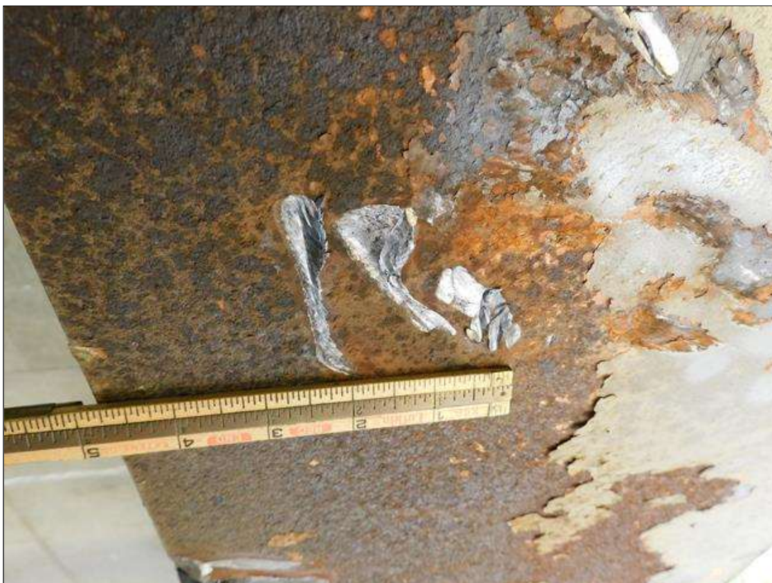
Span 1 Beam 5: IMPACT DAMAGE 4/2022: (3) GOUGES UP TO 2"L x 1/2"W x 1/16"D ON BOTTOM SIDE OF BOTTOM FLANGE - LOCATED 55'-6" FROM END BENT 1 BEARING
