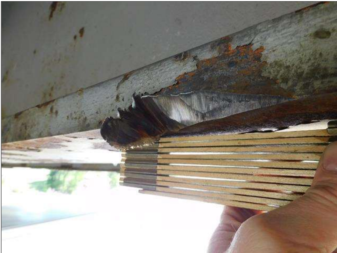
Span 1 Beam 4: IMPACT DAMAGE 4/2022: 3-1/2"L GOUGE UP TO 5/8"D ON NORTH EDGE OF BOTTOM FLANGE - LOCATED 56' FROM END BENT 1 BEARING (PAR)
