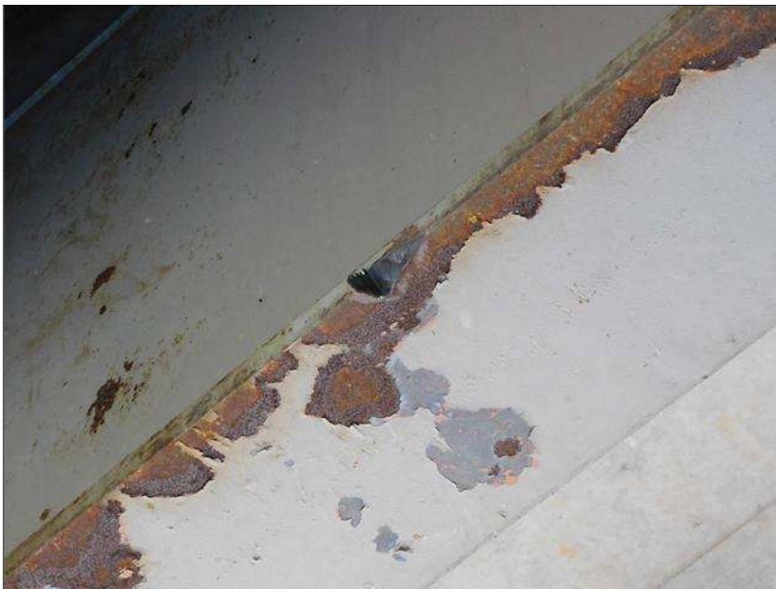
SPAN 1 BEAM 4 - IMPACT DAMAGE OVERVIEW
