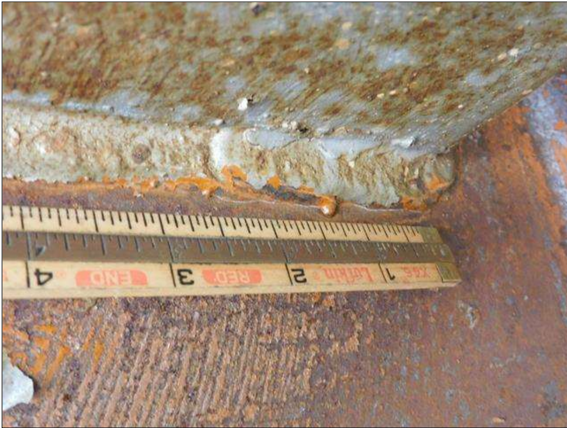
Span 1 Bay 1: IMPACT DAMAGE 4/2022 - INT. DIAPHRAGM 3, BEAM 1 CONNECTION, BOTTOM WELD - 3"L CRACK AT TOE OF WELD (PAR)
