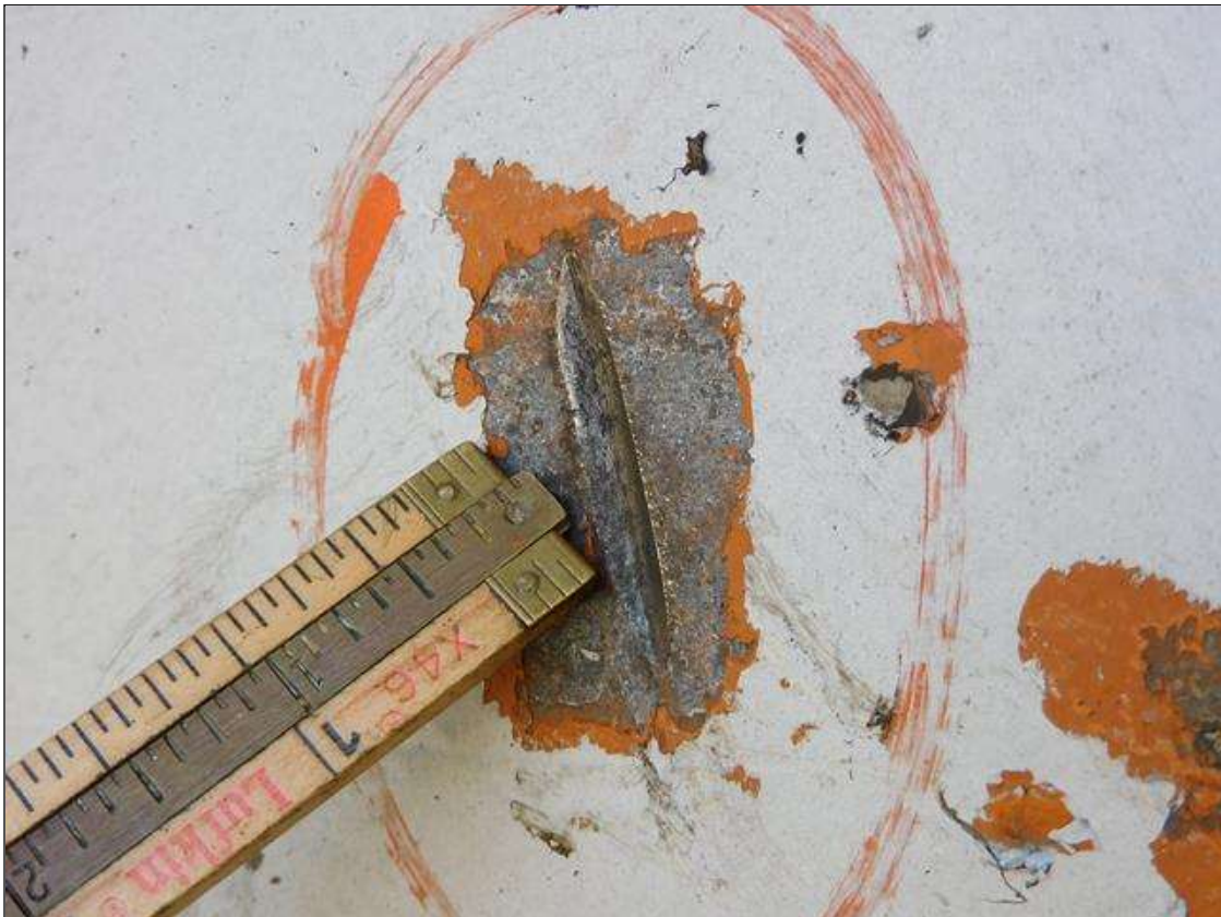
Span 1 Beam 1: IMPACT DAMAGE 4/2022: (3) GOUGES UP TO 2"L x 1/16"D SCATTERED ON BOTTOM 18" OF WEB - LOCATED 55' FROM END BENT 1 BEARING
