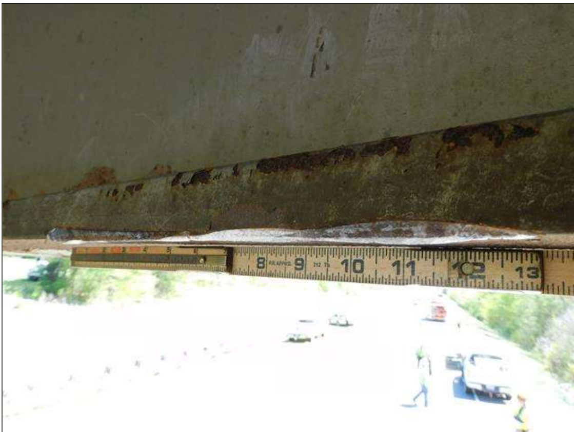
Span 1 Beam 5: IMPACT DAMAGE 4/2022: 13"L x 1/2"W x 1/4"D INDENTION ON NORTH EDGE OF BOTTOM FLANGE AT 57' FROM END BENT 1 BEARING
