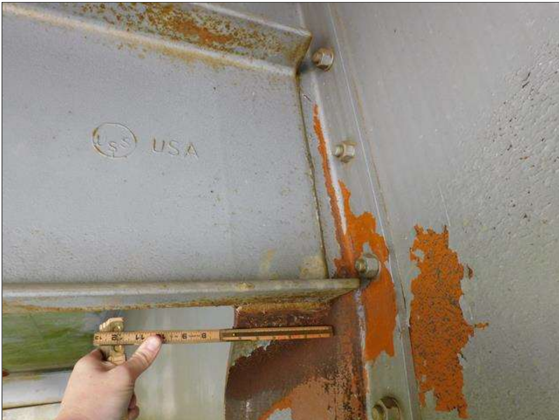
ALT VIEW - Span 1 Bay 1: IMPACT DAMAGE 4/2022 - INT. DIAPHRAGM 2, BEAM 1 CONNECTION, BOTTOM WELD - 4"L CRACK AT TOE OF WELD (PAR)
