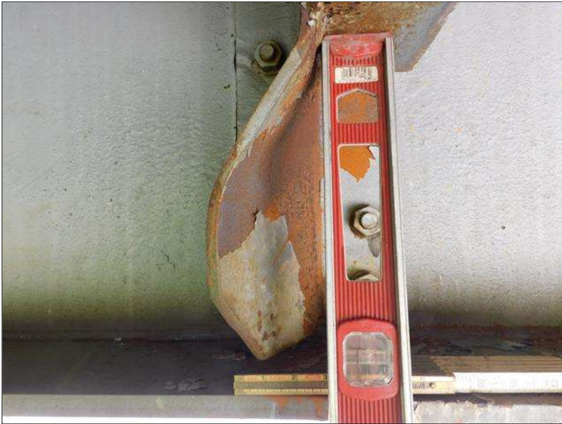
Span 1 Bay 1: IMPACT DAMAGE 4/2022 - INT. DIAPHRAGM 3, BEAM 1 CONNECTION BRACKET - BOTTOM 10" BENT 3-1/2" TO THE WEST (PAR)
