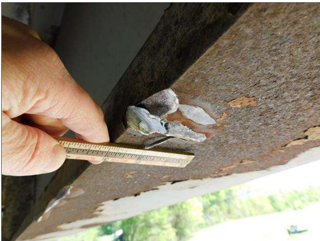
Span 1 Beam 5: IMPACT DAMAGE 4/2022: 2"W x 3"L x 3/8"D GOUGE ON NORTH EDGE OF BOTTOM FLANGE AT 56' FROM END BENT 1 BEARING (PAR)
