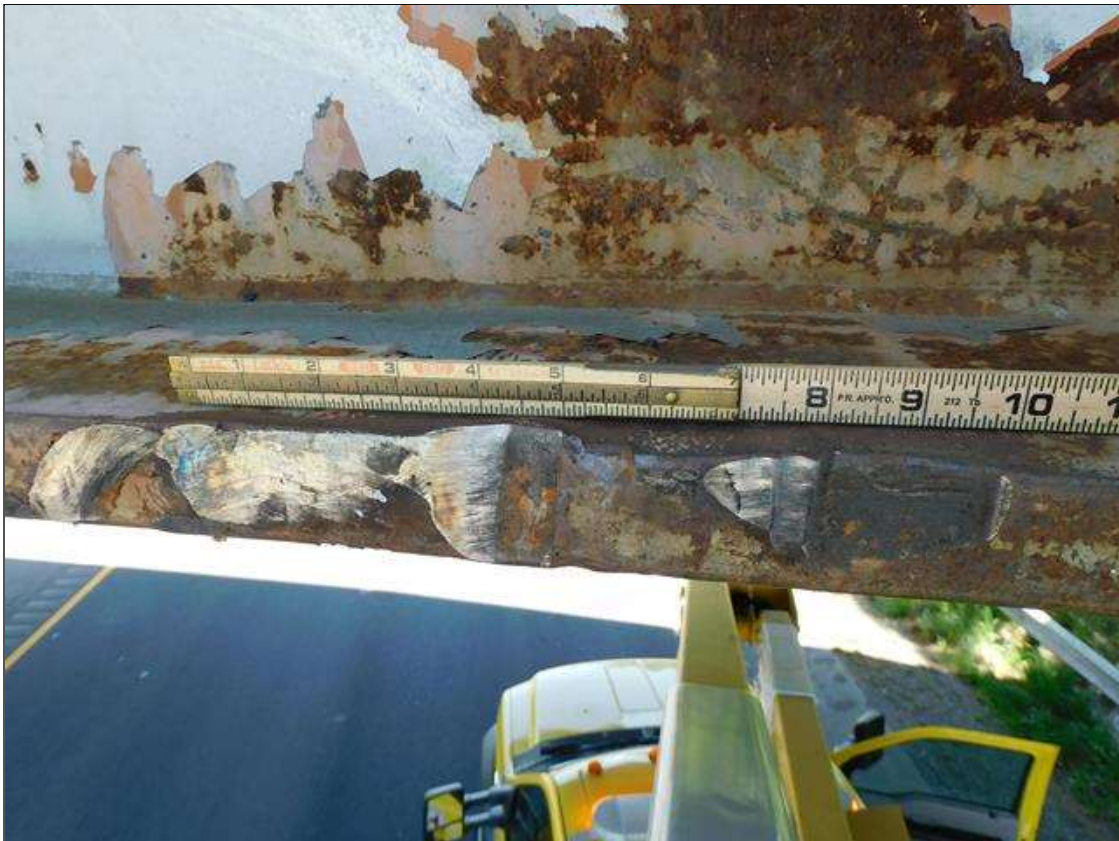
Span 1 Beam 1: IMPACT DAMAGE 4/2022: INDENTIONS UP TO 1-1/2"W x 1/4"D SCATTERED ALONG 10" SECTION OF BOTTOM FLANGE ON NORTH SIDE - LOCATED 56' FROM END BENT 1 BEARING (PAR)
