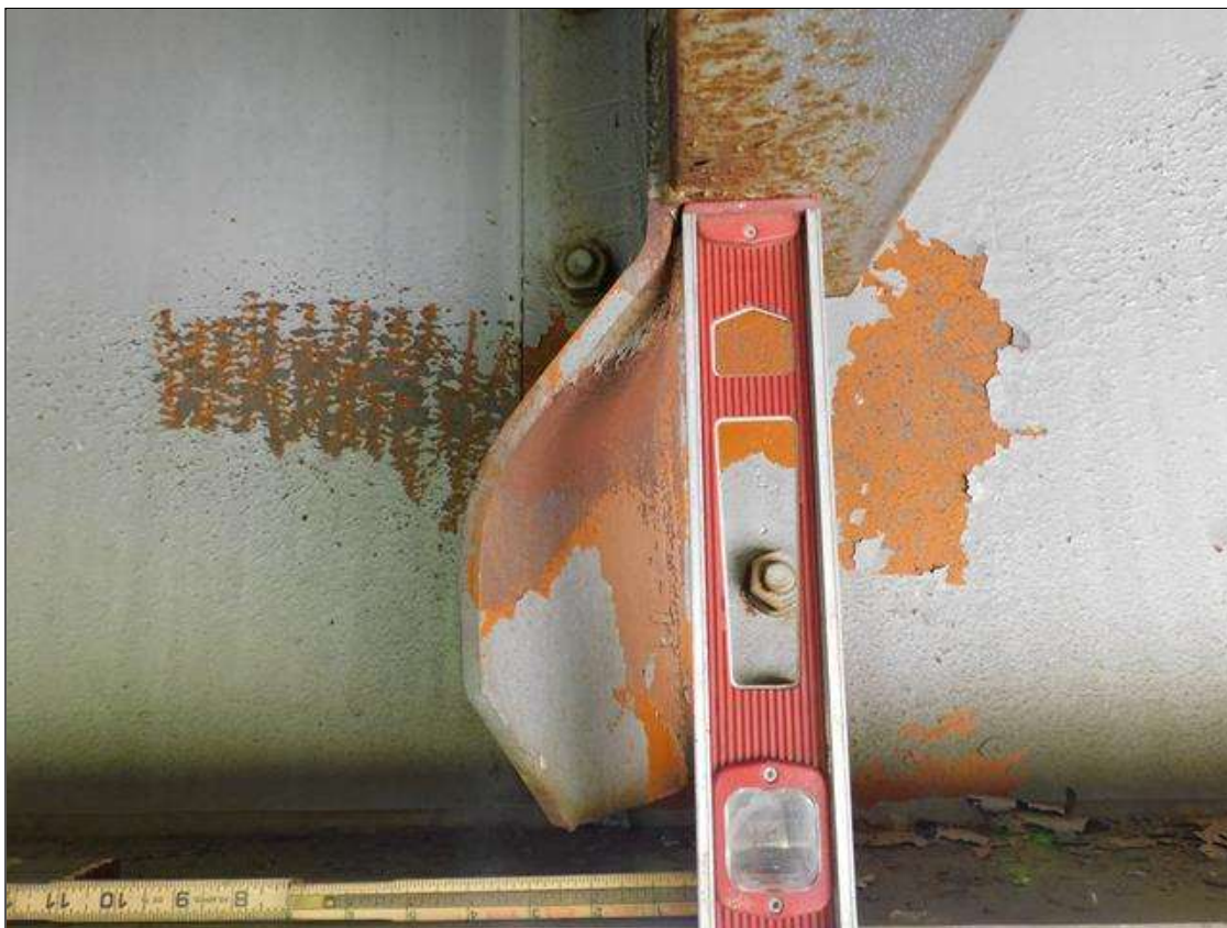
Span 1 Bay 1: IMPACT DAMAGE 4/2022 - INT. DIAPHRAGM 2, BEAM 1 CONNECTION BRACKET - BOTTOM 10" BENT 4" TO THE WEST (PAR)
