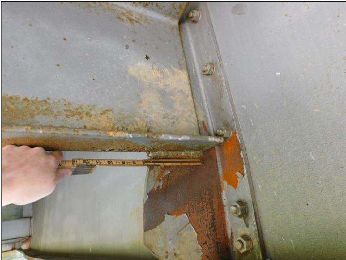
ALT VIEW - Span 1 Bay 1: IMPACT DAMAGE 4/2022 - INT. DIAPHRAGM 3, BEAM 1 CONNECTION, BOTTOM WELD - 3"L CRACK AT TOE OF WELD (PAR)
