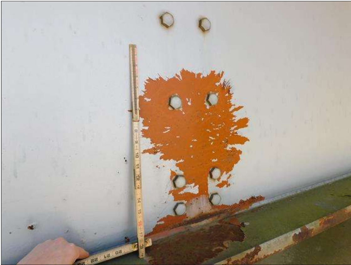
Span 1 Beam 1: IMPACT DAMAGE 4/2022 - 24" DIAMETER SECTION OF WEB DEFLECTED 1-1/4" TO THE NORTH AT INT. DIAPHRAGM 2 CONNECTION (PAR)
