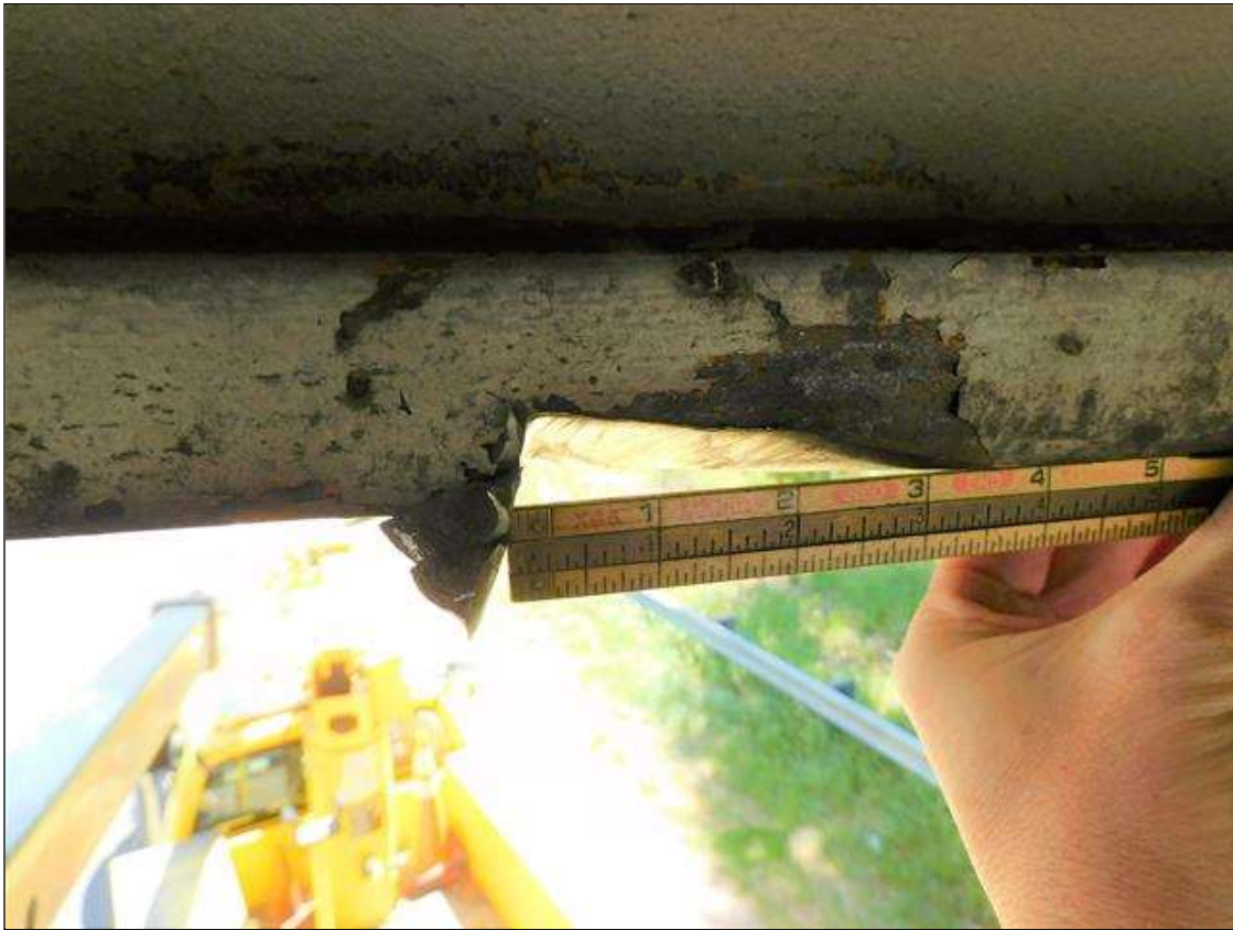
Span 1 Beam 4: IMPACT DAMAGE 4/2022: 3-1/2"L GOUGE UP TO 5/8"D ON NORTH EDGE OF BOTTOM FLANGE - LOCATED 56' FROM END BENT 1 BEARING (PAR)
