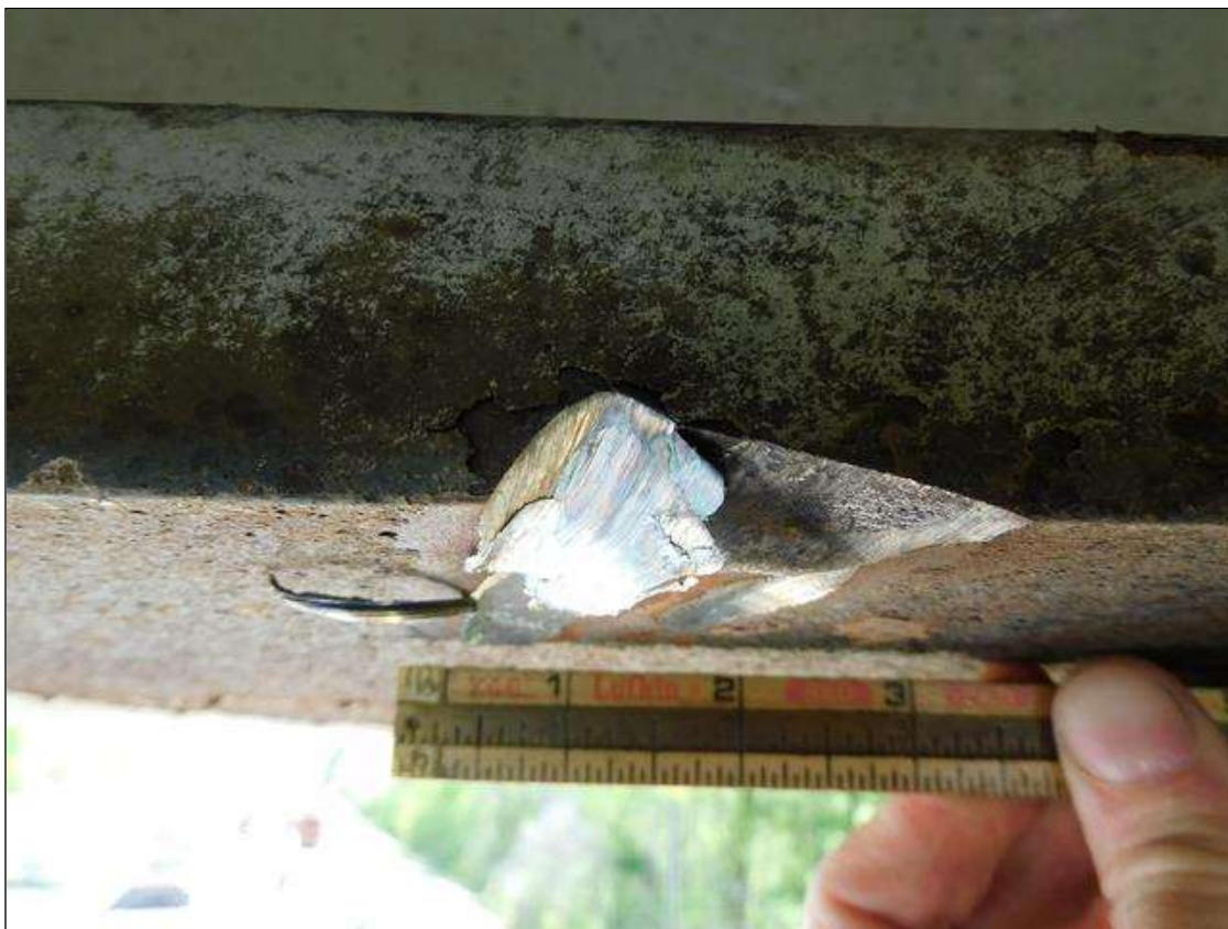
Span 1 Beam 5: IMPACT DAMAGE 4/2022: 2"W x 3"L x 3/8"D GOUGE ON NORTH EDGE OF BOTTOM FLANGE AT 56' FROM END BENT 1 BEARING (PAR)
