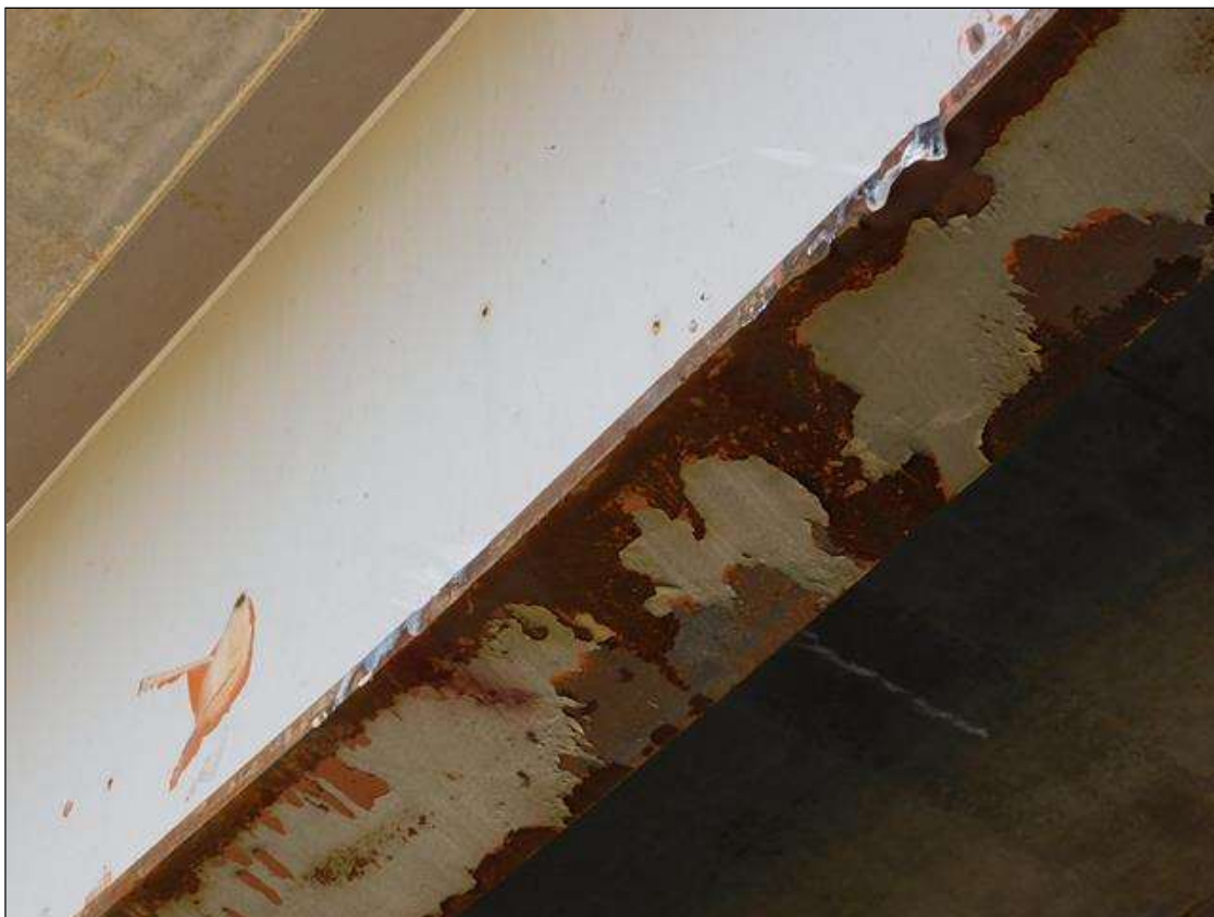
SPAN 1 BEAM 1 - IMPACT DAMAGE OVERVIEW
