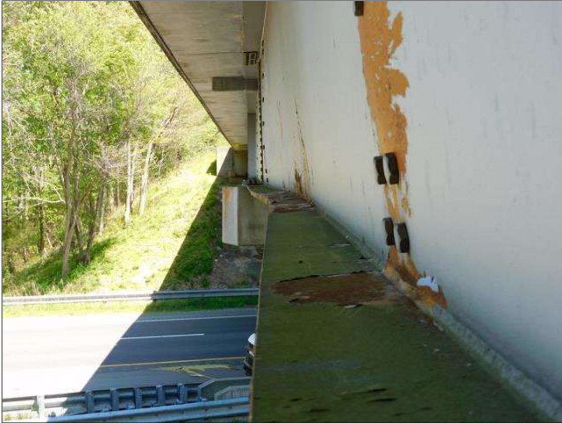
Span 1 Beam 1: IMPACT DAMAGE 4/2022: 23LF OF BEAM OUT OF PLUMB TO THE SOUTH UP TO 4-3/4" - MAX DEFLECTION AT 55' FROM END BENT 1 BEARING - SECTION LOCATED BETWEEN INT. DIAPHRAGMS 2 AND 3 (PAR)
