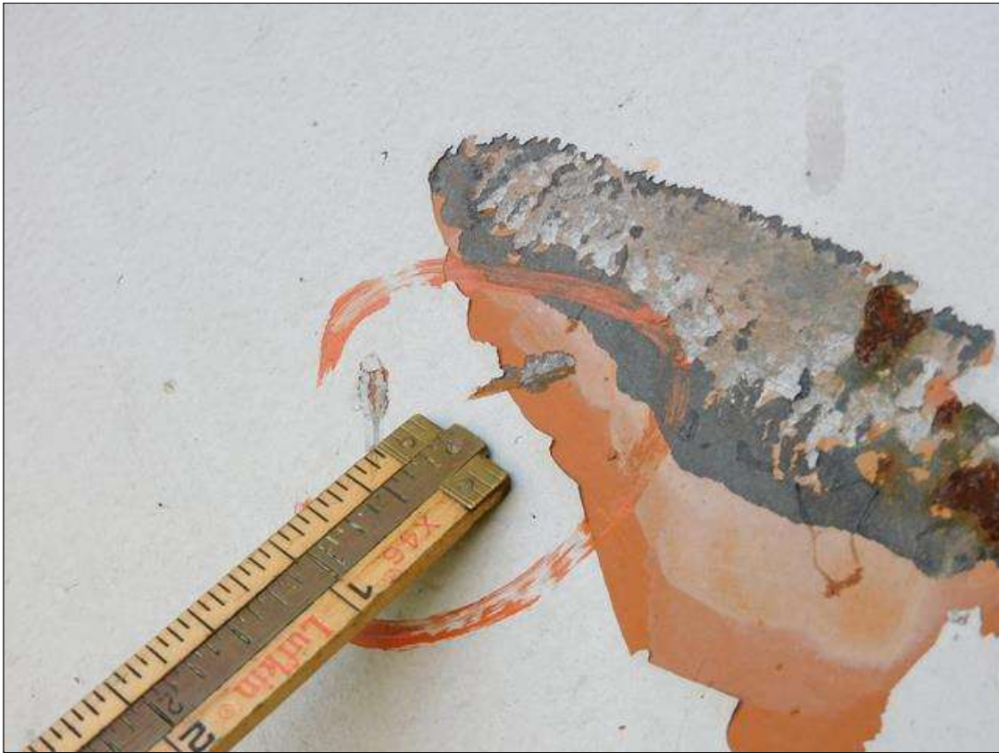
Span 1 Beam 1: IMPACT DAMAGE 4/2022: (3) GOUGES UP TO 2"L x 1/16"D SCATTERED ON BOTTOM 18" OF WEB - LOCATED 55' FROM END BENT 1 BEARING
