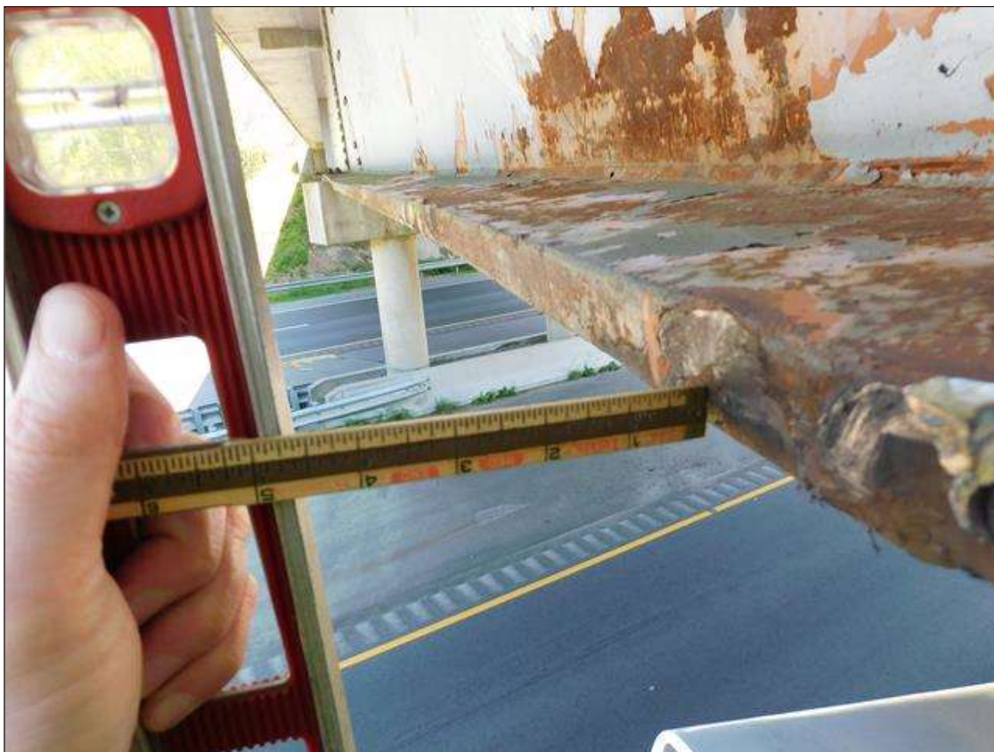
Span 1 Beam 1: IMPACT DAMAGE 4/2022: 23LF OF BEAM OUT OF PLUMB TO THE SOUTH UP TO 4-3/4" - MAX DEFLECTION AT 55' FROM END BENT 1 BEARING - SECTION LOCATED BETWEEN INT. DIAPHRAGMS 2 AND 3 (PAR)
