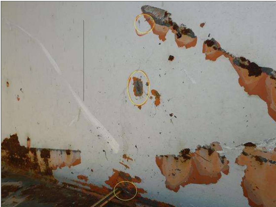
Span 1 Beam 1: IMPACT DAMAGE 4/2022: (3) GOUGES UP TO 2"L x 1/16"D SCATTERED ON BOTTOM 18" OF WEB - LOCATED 55' FROM END BENT 1 BEARING
